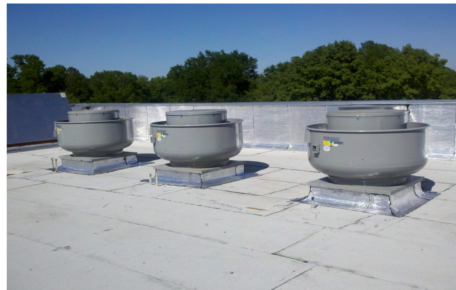
Kitchen exhaust outlets on the Broadhead Center roof
